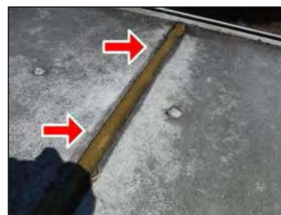
Gaps at seams
