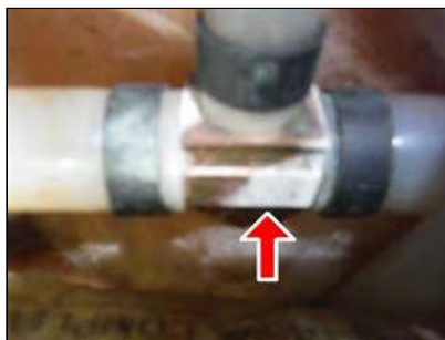
Corrosion on exterior of fitting
