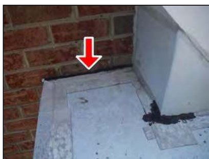
No flashing to brickwork
